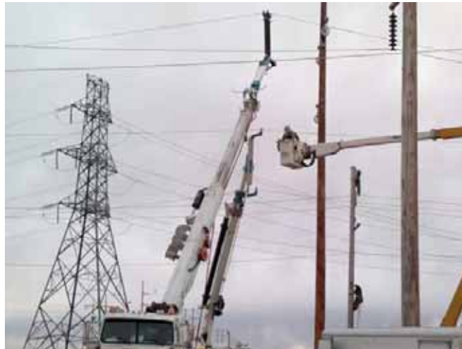
Figure 4.3 A photograph showing live line crews working on a 138 kV energized line at a construction site near Brooks, Alberta. Another worker is seen to climb a pole with a risk of fall.
