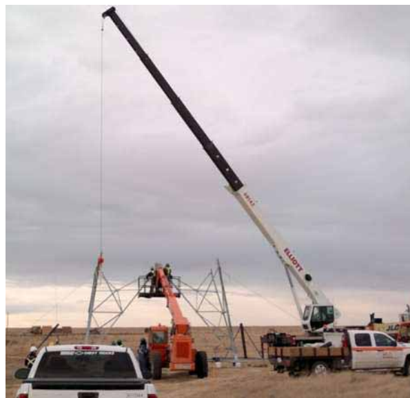
Figure 4.7 A photograph showing workers at risk of fall and of being hit by falling objects
